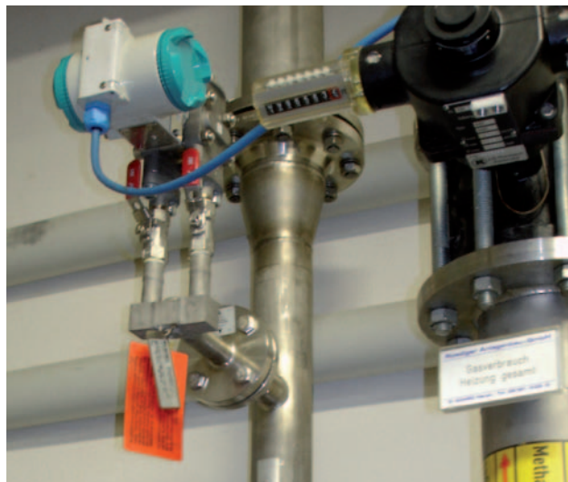
Deployment of deltaflow for biogas flow metering.
